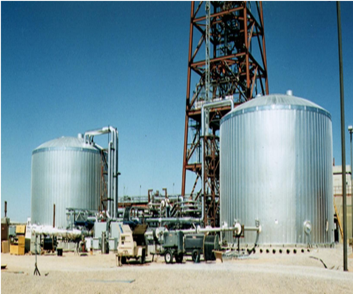
Figure 2.3.2: Solar two central receiver tower plant's TES system consist of cold and hot tanks from left hand side of the image respectively. Solar two TES tanks operate on binary solar salt. The power tower is seen in between the two tanks [55].
