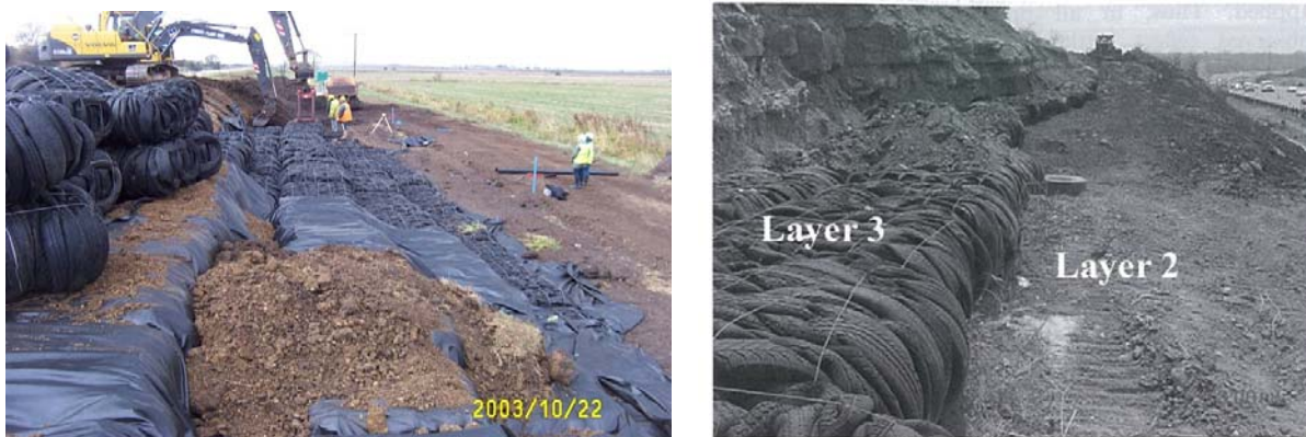
Figure 1: Tyre bales as embankment fill (a) Application in Flood Embankment (b) Highway Embankment.
