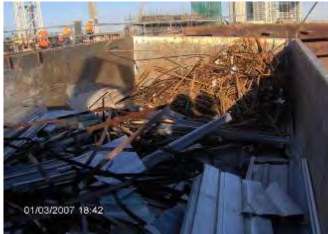
Figure 6.8: Steel correctly disposed of in the appropriate bin
