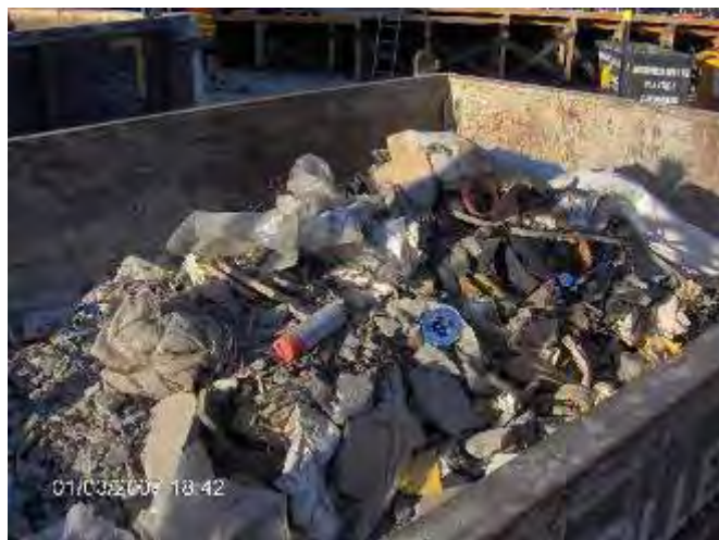
Figure 6.9: Incorrect disposal of other waste in Concrete bin
