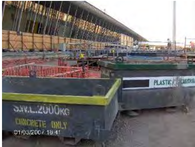
Figure 6.10: Labelled bins at the MCC site
