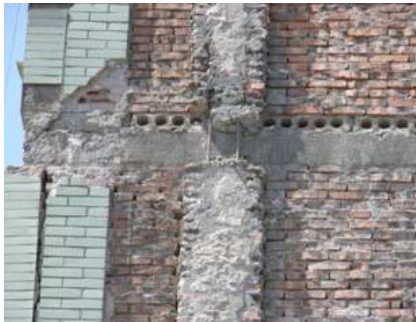
Figure 1. Poor beam-joint connection
