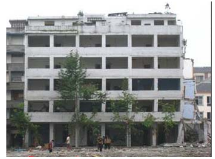
Figure 3. Soft storey damage of second storey with drift of about 5.6% in Dujiangyan
